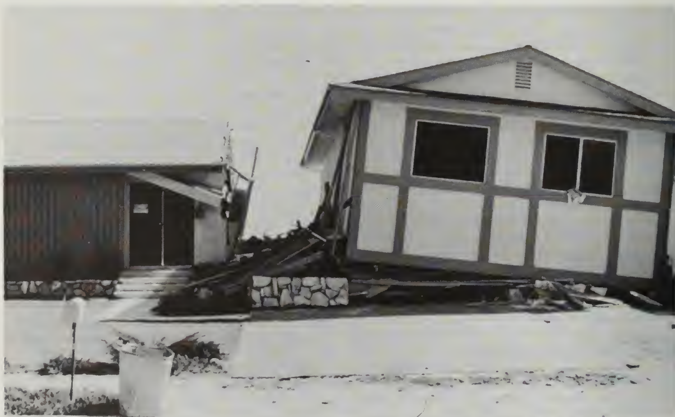
Residence torn apart by fault rupture during the 1971 San Fernando earthquake. Such occurrences led to the Alquist-Priolo Special Studies Zone Act of 1972, which introduced the concept of special studies zones to prevent certain types of development across active faults. Photo from University of Southern California, Department of Geological Sciences.
